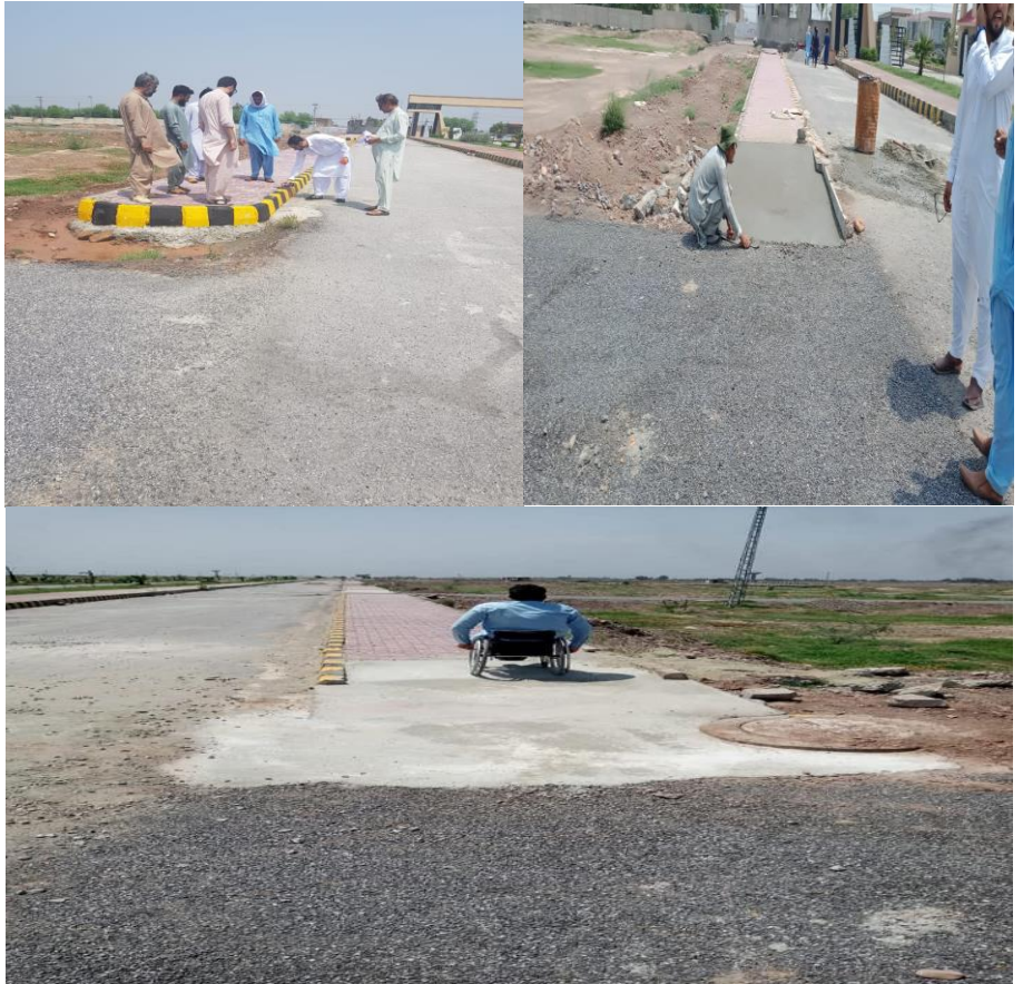
Reconstruction of Pathways to make it accessible for physical challenged people in Provincial Housing Authority Jalozai scheme Khyber Pakhtunkhwa.
